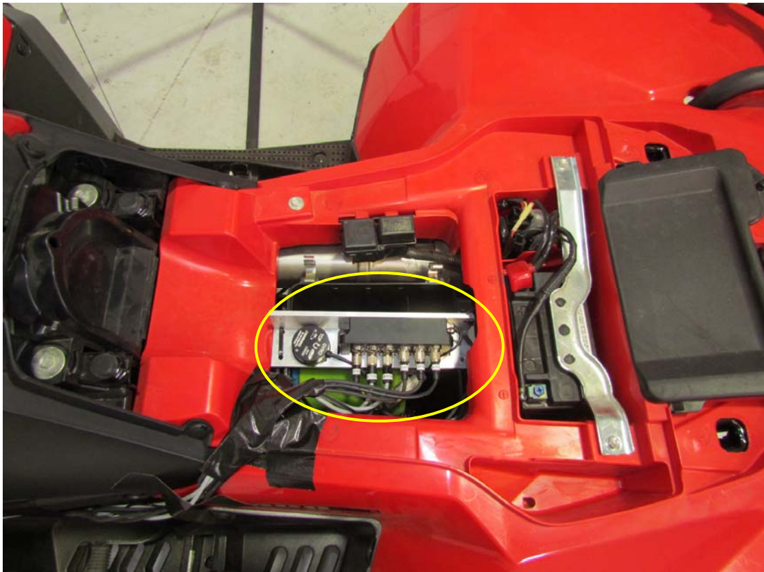
Data acquisition system, accelerometers and rate gyro installed close to COG (typical installation)
